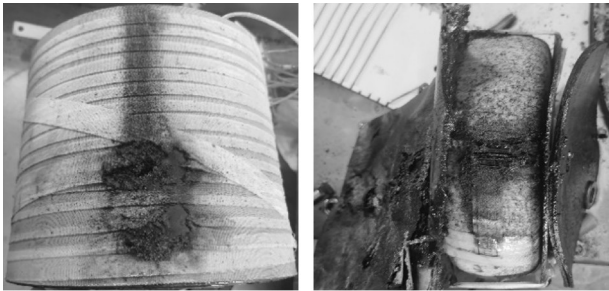
图5 一次绕组及速饱和电抗器击穿部位 Fig. 5 Breakdown position of primary winding and fast saturation reactor
